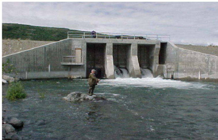
Aishihik Control Structure – Aishihik, Yukon
