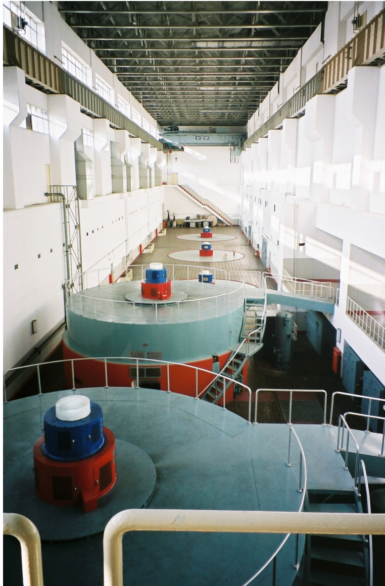
Photo.1: Nam Ngum 1 Power Station
